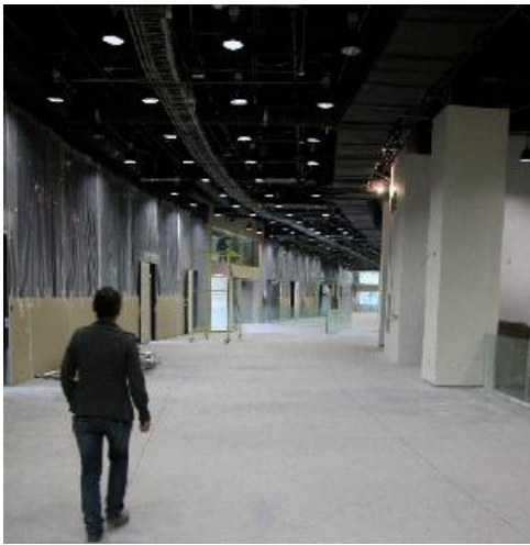
UNDER CONSTRUCTION Q2 2010 Tumo, Armenia. Epygi. 60pc DIDIO 7017
